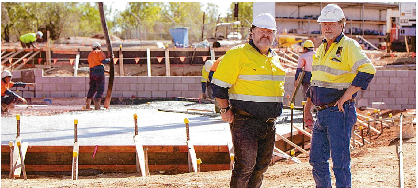
Power and Water Project Manager Liam Early and Yingwati Civil Construction Manager Theo Rapp on site
