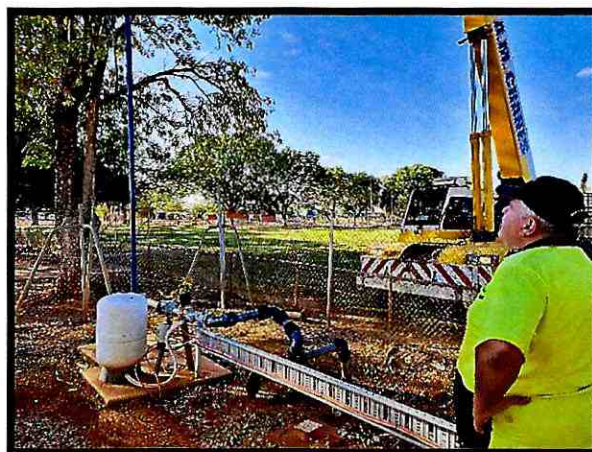
KTC staff member spotting the Contractor while bore repairs taking place at the Sportsgrounds
