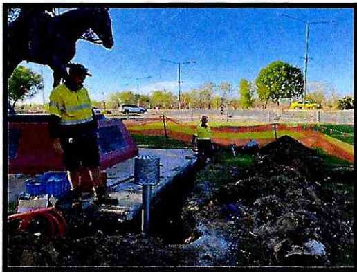
KTC staff digging a trench at the Sabu Sing – Stockmen’s Pioneer Memorial
